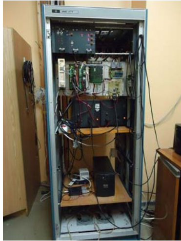
Figure 17. The control panel. From top to bottom: power supply; JVL driver SMC 35 SMD41B3 (green color); GPS Garmin 35 LP.
